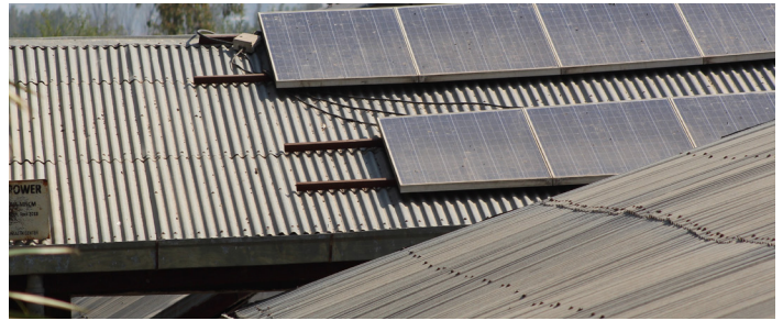
A solar power system that was installed at one of the health facilities supported by the project.
