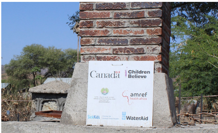
Incinerator built in the Artuma Health Centre, Artuma Fursi district.
